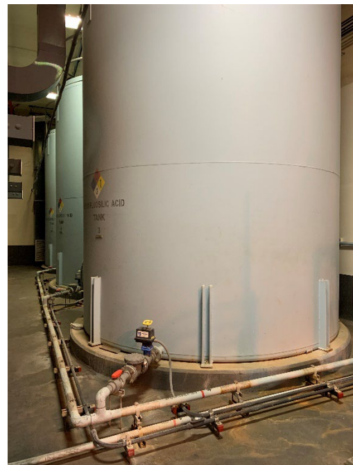
Fluoride Tanks and Piping
